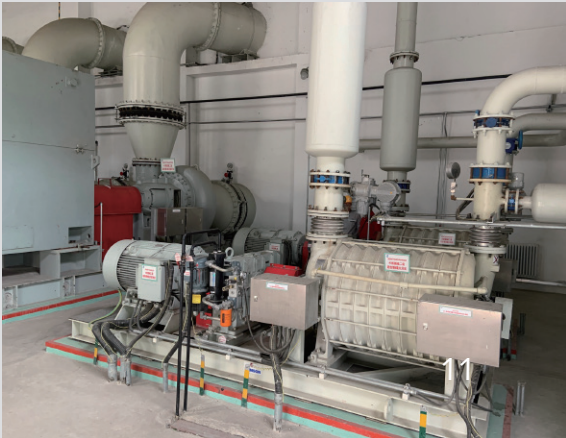
莱州电厂 Laizhou Power Plant
